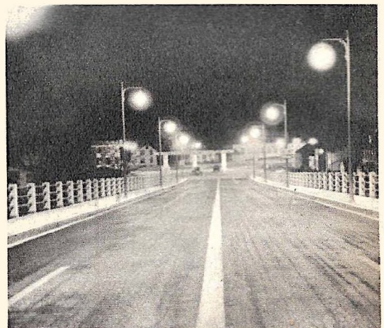
Night scene on the new Delaware River toll bridge at Easton, Pa., showing the glareless and shadowless vapor lamps used.
