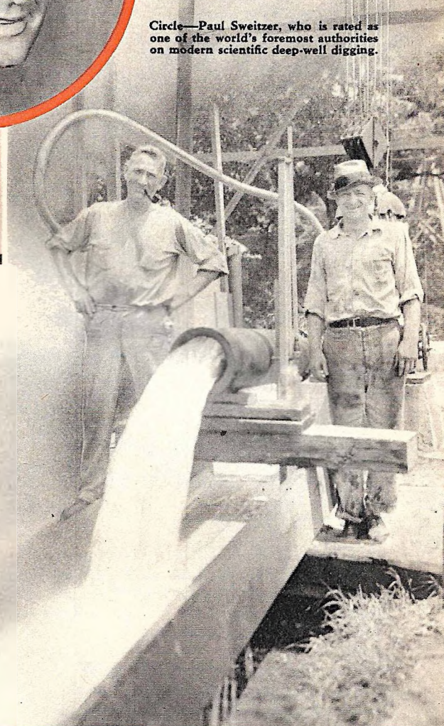
No wonder Mr. Sweitzer (wearing hat) and his assistant are smiling—the water pouring from the pipe during a test indicated that the new well in the background would yield two million gallons daily.
